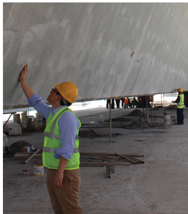
The bridge spans are quality-assured before being lifted to the storage facility for setting.
