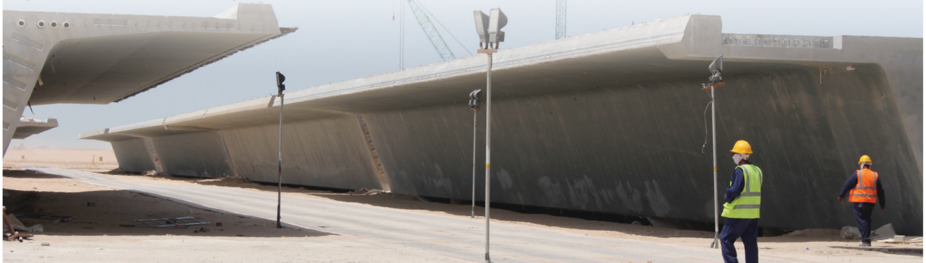
The giant bridge spans in the storage facility in the desert where they are left to set prior to offshore transport and installation.
