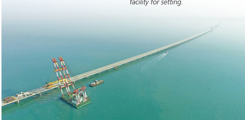
Floating cranes are lifting bridge pillars and bridge spans in place in the bay.
