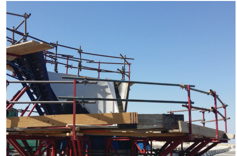
Steel shutterings are lined with Formtex® – it is important that the cloth follows the curves of the mould.
