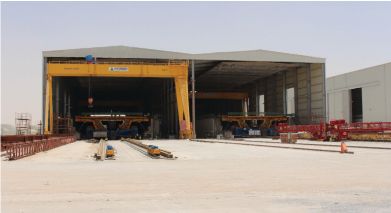
Special casting hangars were built for the construction of the 60 x 25 x 7 m spans.
