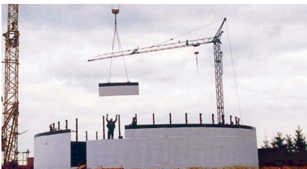
Figure 2. An element lined with Formtex® is hoist into place by a tower crane.
