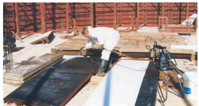
Figure 3. Glue is sprayed onto a formwork element and a length of Formtex® is unrolled.
